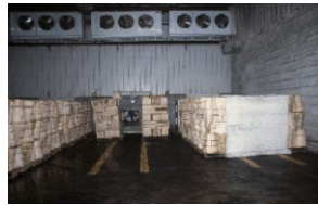
Figure 47. Commercial forced air cooling system.
