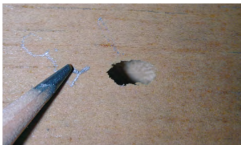
Wood-boring beetle exit hole
