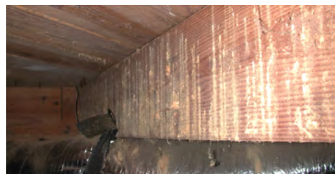
Visual evidence (frass streaming from exit holes) of an active anobiid powderpost beetle infestation in a crawlspace joist
