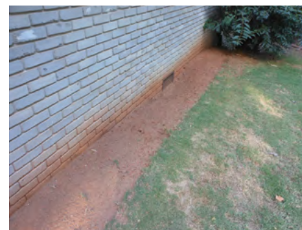
Figure 7. The area next to foundation walls should be kept free of vegetation.
