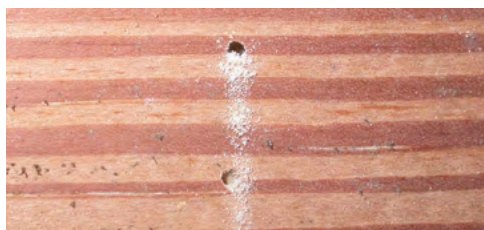
Anobiid powderpost beetle exit holes in an infested crawlspace joist
