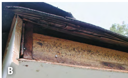
Figure 5. The structure itself is comprised of an almost endless series of voids and other potential harborage sites, such as (A) crawlspaces, and (B) the attic area behind fascia boards, where smokybrown cockroaches were living (the dark stippling is cockroach frass).
