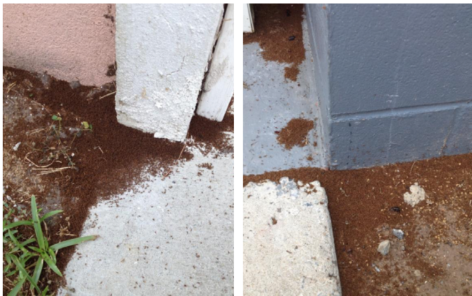
Figure 2. Dead tawny crazy ants commonly collect in corners and along walls on the outside of infested structures, a telltale sign of infestation.
