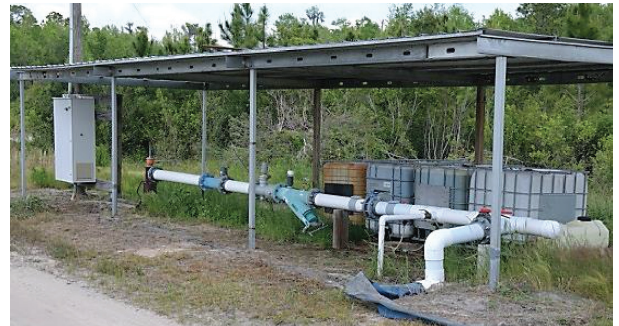
Figure 10. Well head, backflow, flow meter, filter, venturi, chemical totes, and electrical control panel under a lean-to structure.
