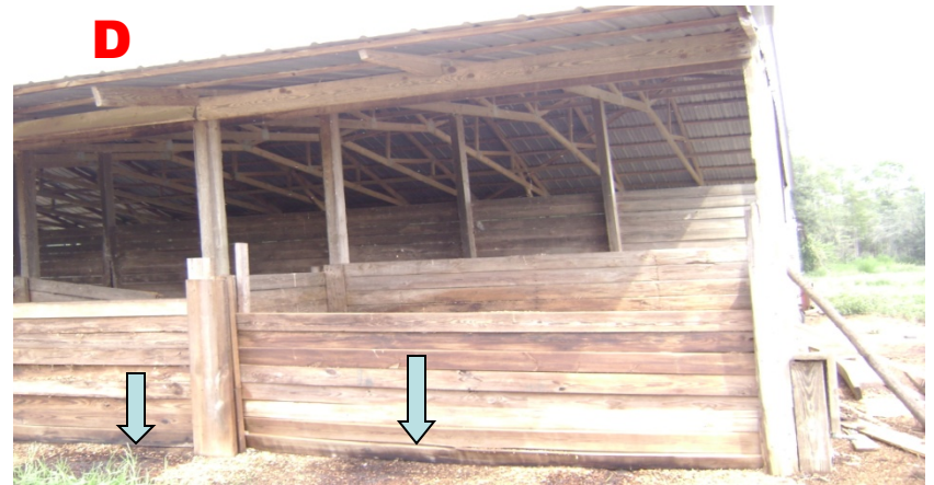
Leaching from the pile can cause odors and flies.
